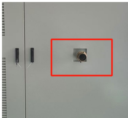
Figure 11-10 Ports on a cabinet fire hose
