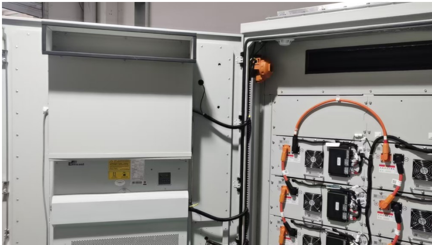
Figure 11-9 Air intake air outlet of the cabinet
